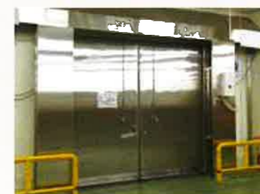
Cold storage Inside -25°C / Outside 5°C Size: 3,000mm (h) x 2,600mm (w) Door opening by Pull switch
