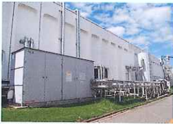
● Carbonated beverages cooling system
